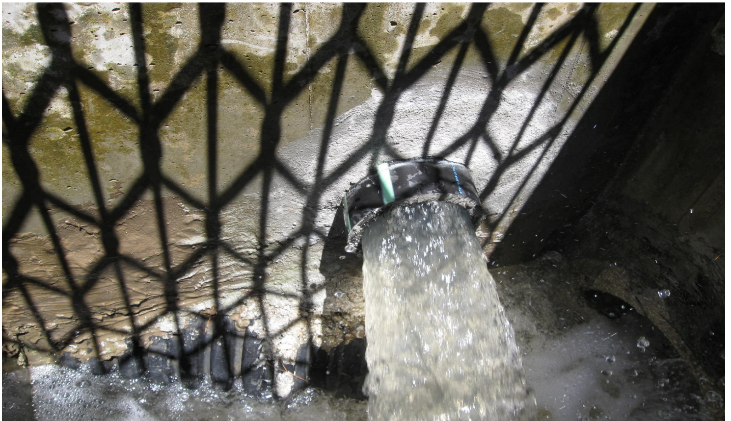
Pump Discharge in box at SW 47th Ave and I-75
